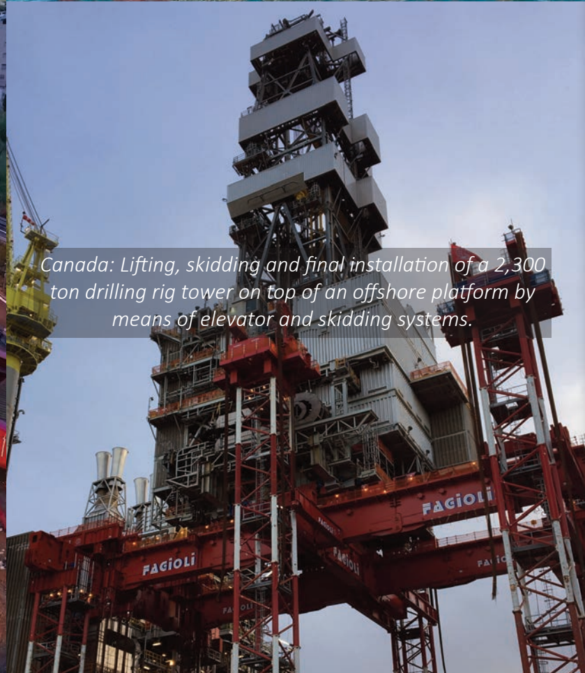
Siffredi bridge, Genoa: Transport and installation of a 406 ton bridge by means of Fagioli SPMTs, Jack-up system, Gantry Cranes and Rollers.
